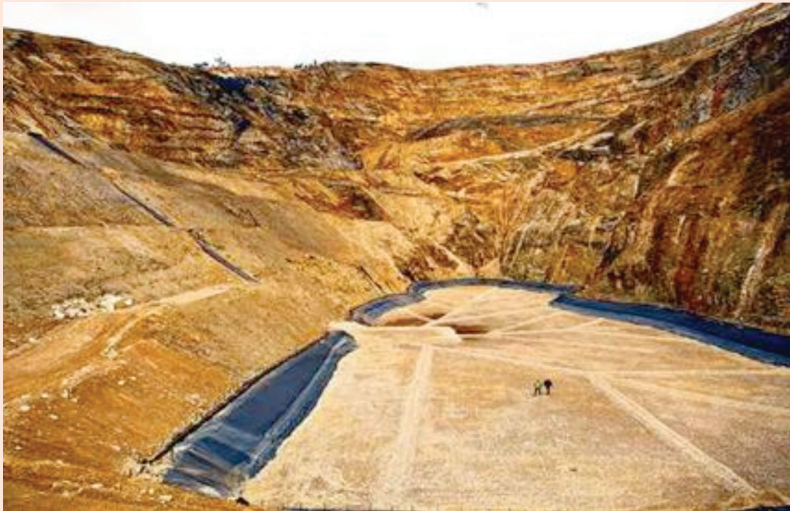
Early days in the bioreactor's life—the base liner in place in the open cut.
