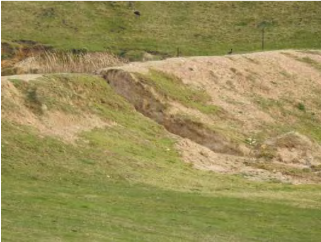
Figure 32: Impacts of dispersive soils and inappropriate clays on dam construction at Glenaladale
