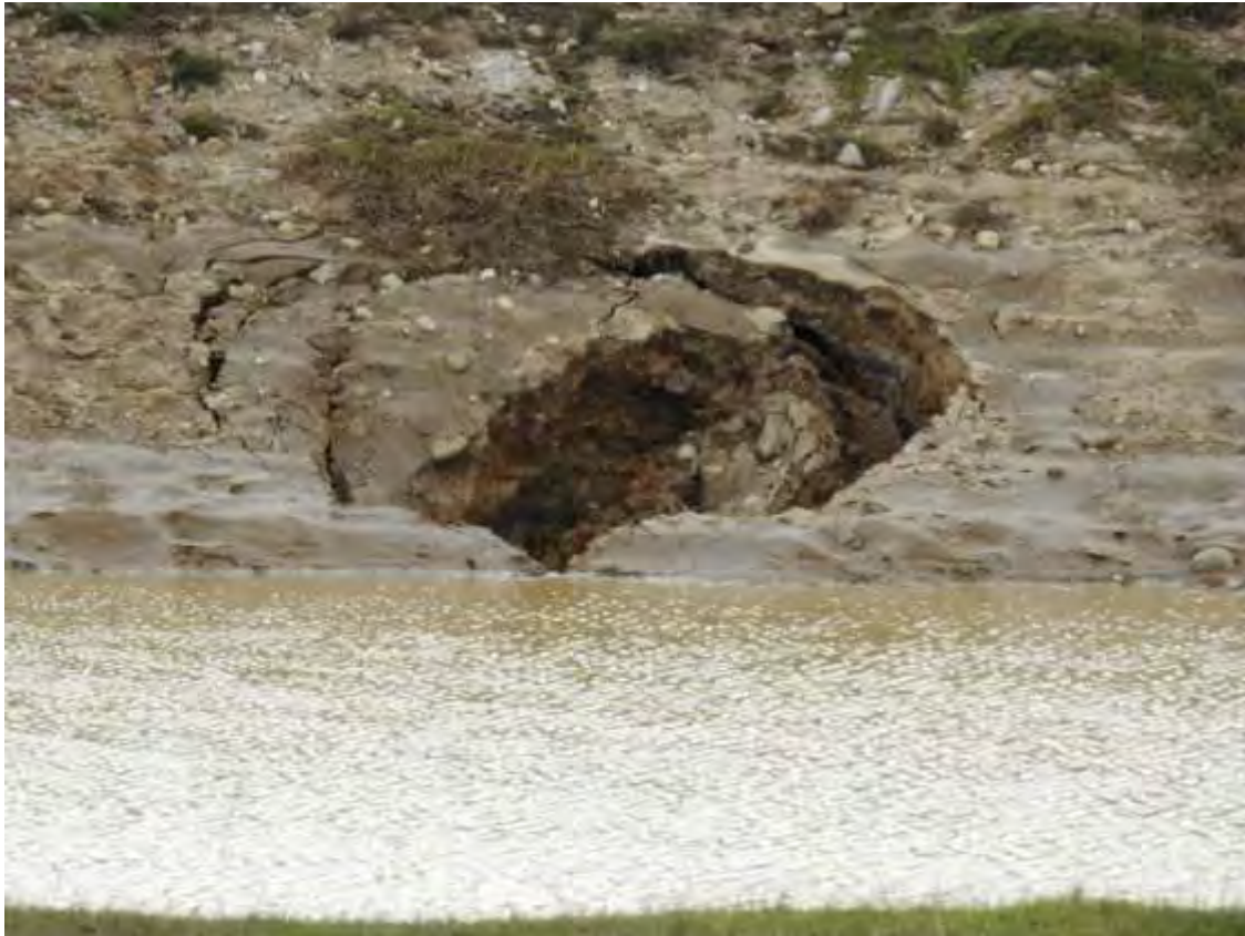
Figure 33: Subsidence that occurs when inappropriate clays are used in dams
