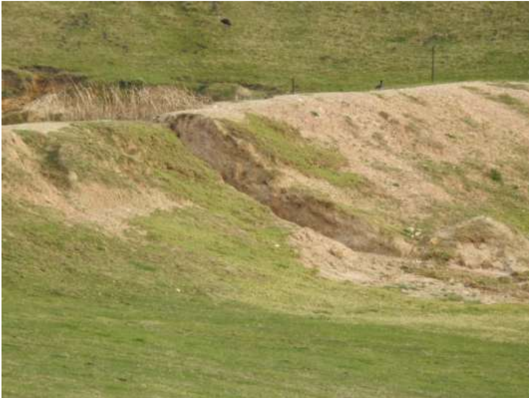
Figure 32: Impacts of dispersive soils and inappropriate clays on dam construction at Glenaladale
