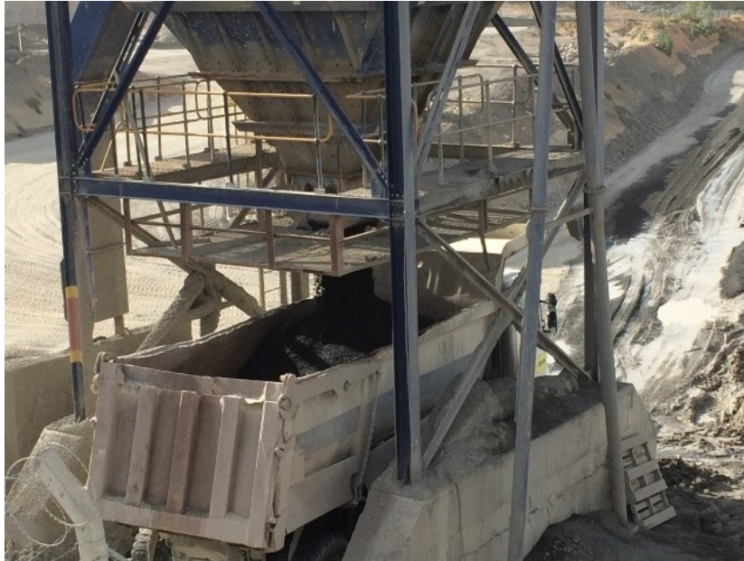
Figure 15 Solid discharge into truck after mixing underflow of hydrocyclone and solid of centrifuge, no addition of any surcharge material required
