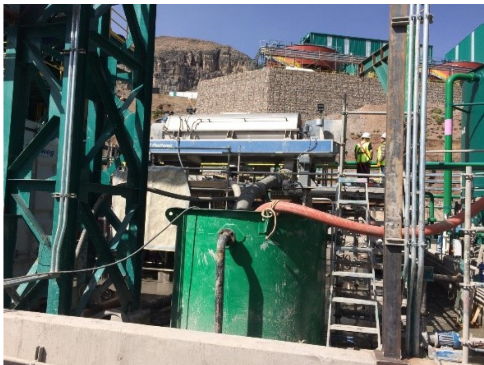
Figure 8 Centrifuge installation at Buenaventura Tambomayo mine
