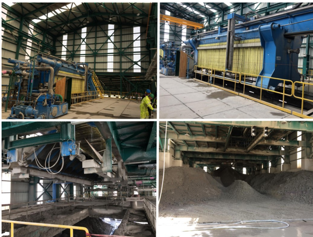
Figure 7 Multi-storey filter press building at Buenaventura's Tambomayo mine
