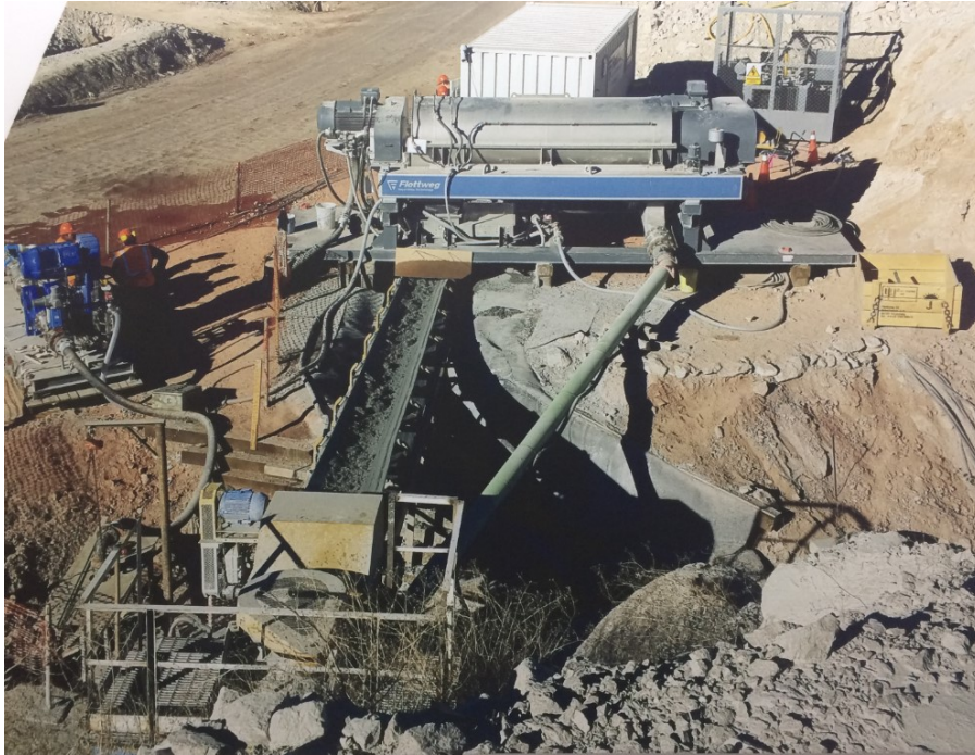
Figure 18 Centrifuge installation at Cuajone mine
