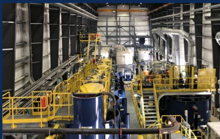
Harte Gold processing plant
