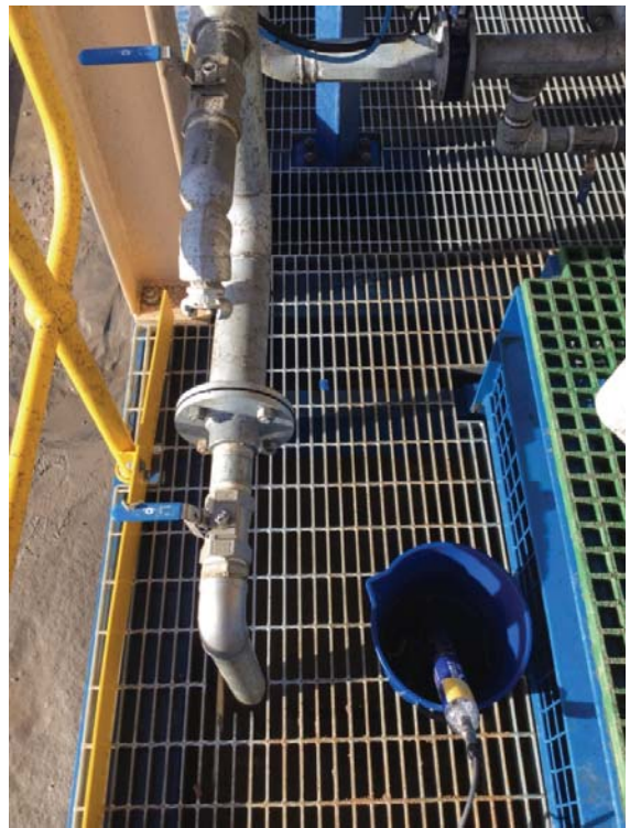
Description: Purge 2 buckets MINIMUM to clear the process water pipe.
