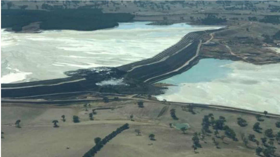
Figure 14: Upstream failure - Cadia dam Sydney Morning Herald March 2018
